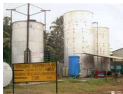
Effluent Treatment Plant
